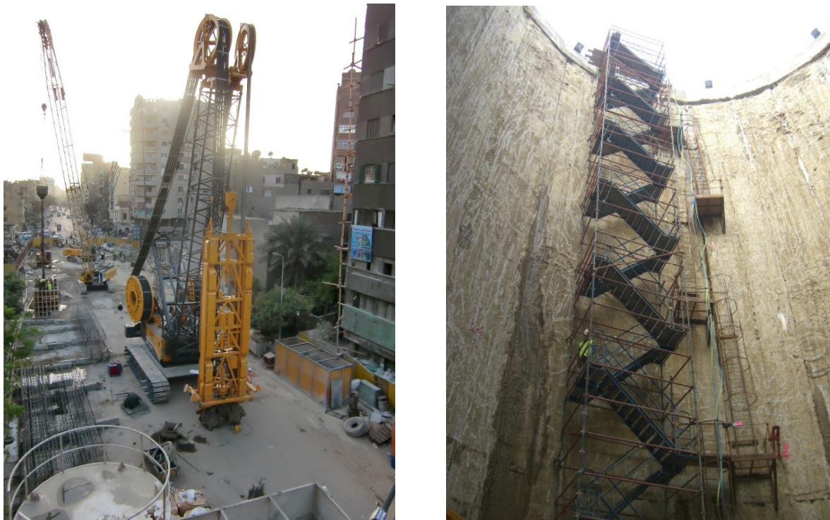
Figure 4: Site impressions of the rescue shaft before the start and after finish of construction
