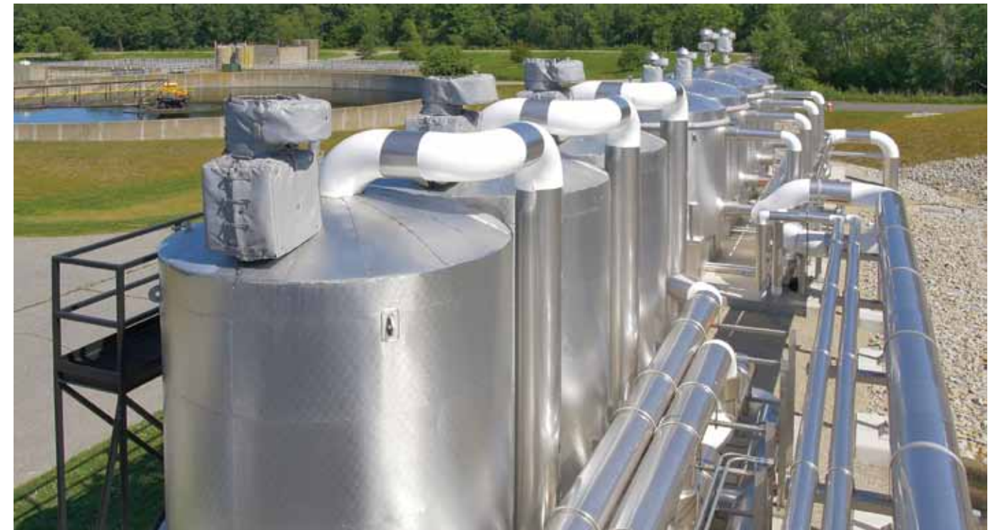
Biogas is treated for H 2 S and siloxane removal prior to beneficial use
