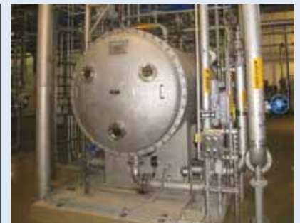
An ozone generator installed at the Shoal Creek Filter Plant. Photo courtesy of Gwinnett County Department of Water Resources
